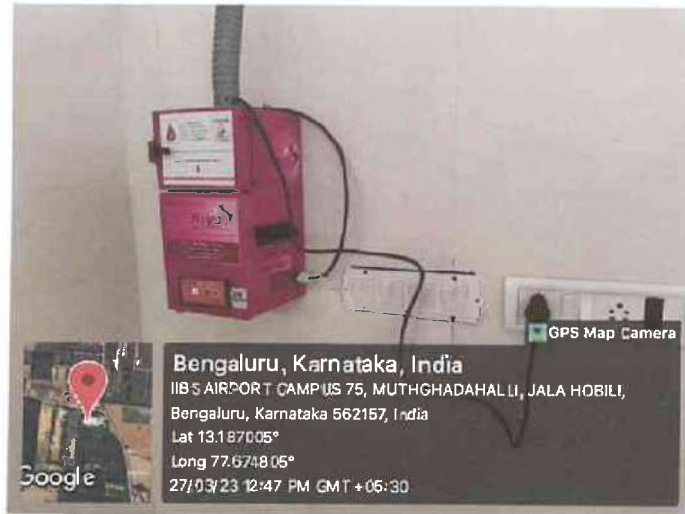
Sanitary Napkin Incinerator
