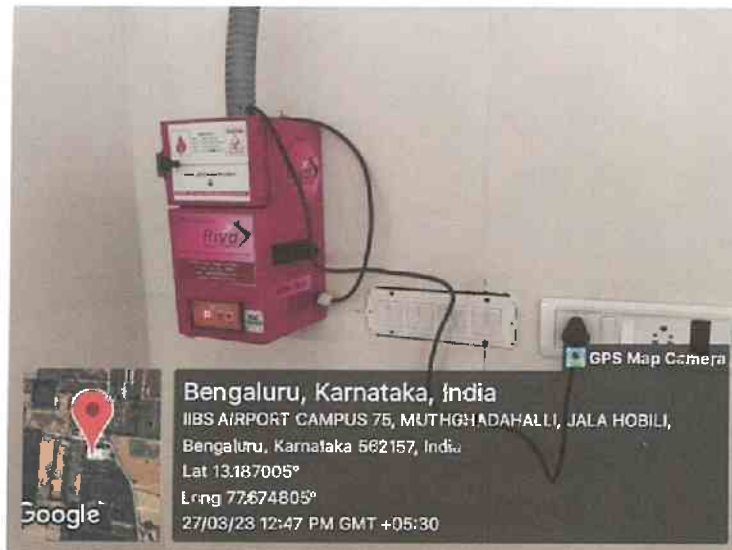
Sanitary Napkin Incinerator
